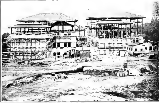
The Carnegie Technical Schools. Two new buildings in the group for the School of Applied Science. To be ready in October. Photograph by S. L. Haas
