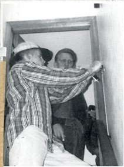
Testing his knowledge of circuitry, Jody Wilson works at the receptacle box. Left Center: Brian Hawkins, Tom Edwards, Jody Wilson, and Brian Wooten make progress on the lighting system of the Mt. Airy Church of God.
