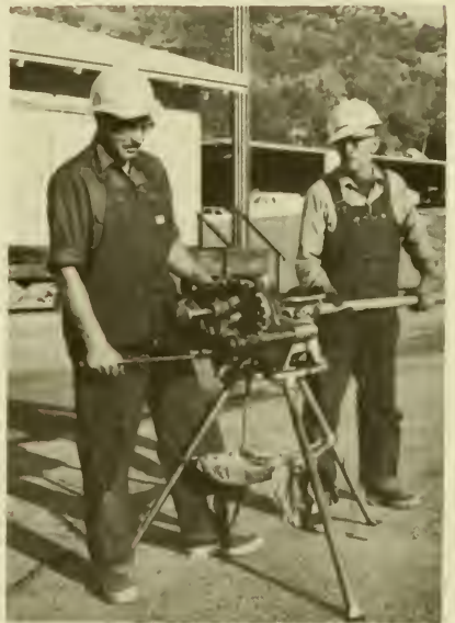
MOCCASIN CORP. YARD Pipe Threading ERVIN JOHNSON (L), Plumber BILL STEELY, Plumber
