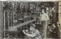
A Real Switchboard in the Coyne Shops
