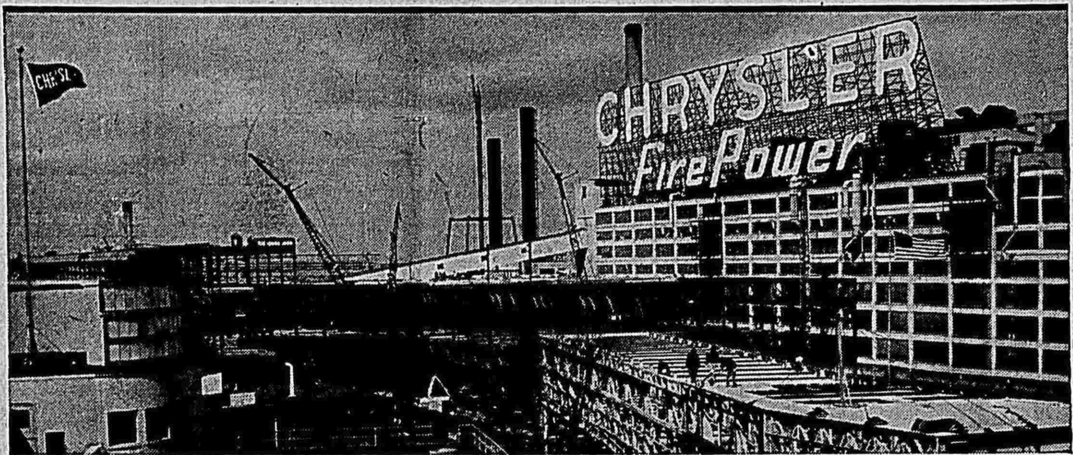
UP GOES CHRYSLER'S PRODUCTION MORE THAN 40% Here you see construction work proceeding on the new Chrysler production facilities which will add 667,000 square feet of floor space... including a 14-mile long continuous conveyor system, longest in the industry.
