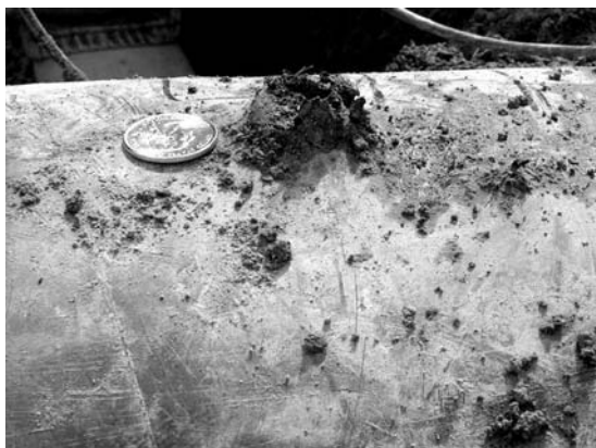
Figure 3-56: Pipeline Anomaly Due to AC Corrosion (Before Cleaning)
