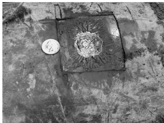
Figure 3-57: Pipeline Anomaly Due to AC Corrosion (After Cleaning)
