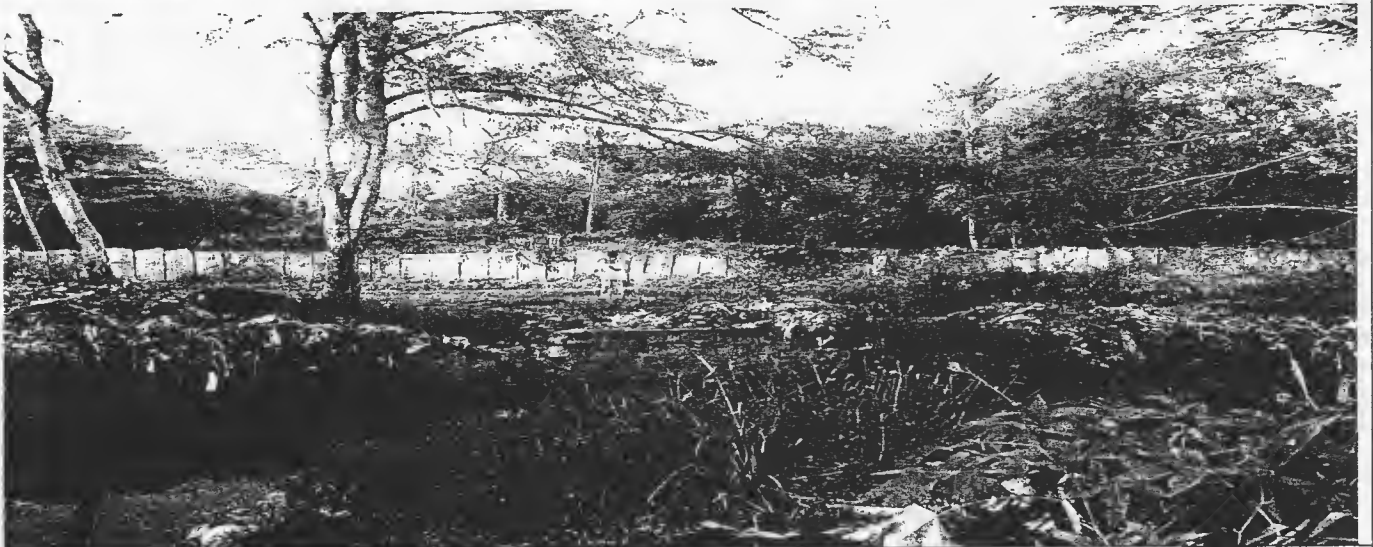
VIEW OF THE WASTEWATER FLOW IN DAMAGED DIVERSION DRAIN FROM WESTERN SIDE OF BHADRAPPA LAYOUT
