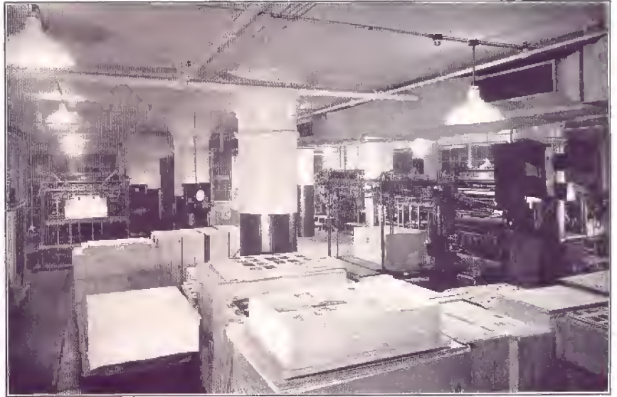
Air conditioned printing-press room of Edward Stern and Co., Philadelphia, equipped in 1932. Chas. S. Leopold, consulting engineer.
