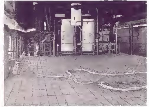
Ice tank with accumulator and set of dehydrators for drying air in the medium-pressure system.
