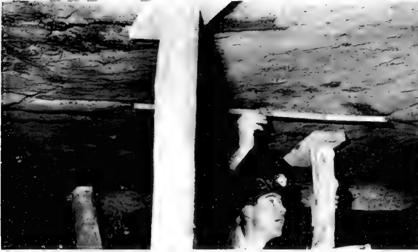
Measuring the distance between the dinosaur footprints in the ceiling of Westvale Colliery, Rosewood, southeast Queensland.
