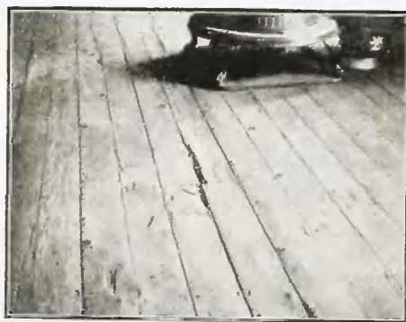
FIGURE 62.—Floor full of cracks.
