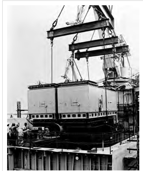
A heavy lift lowers the main propulsion module into the hull of USS Bunker Hill (CG-52) during construction at Ingalls Shipbuilding. The module consists of two General Electric LM2500 gas turbine engines and a Westinghouse gear reduction unit.
