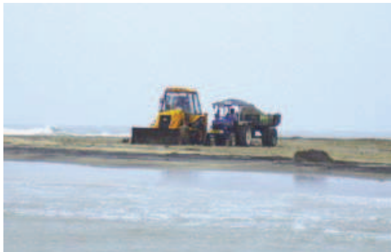
PLATE 12 Sand mining right on the coast in Kallar river –Nagapattinam district Photo by Mr. Mathivanan –TNEC
