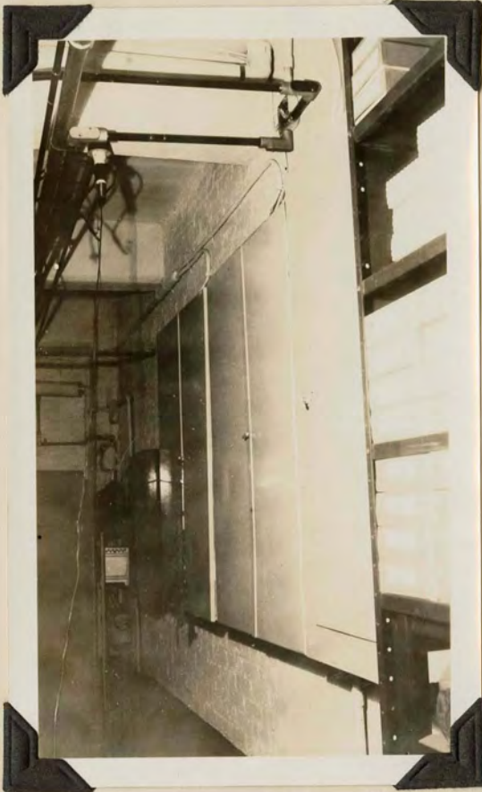
Distributing Frames and Fuse Panel
