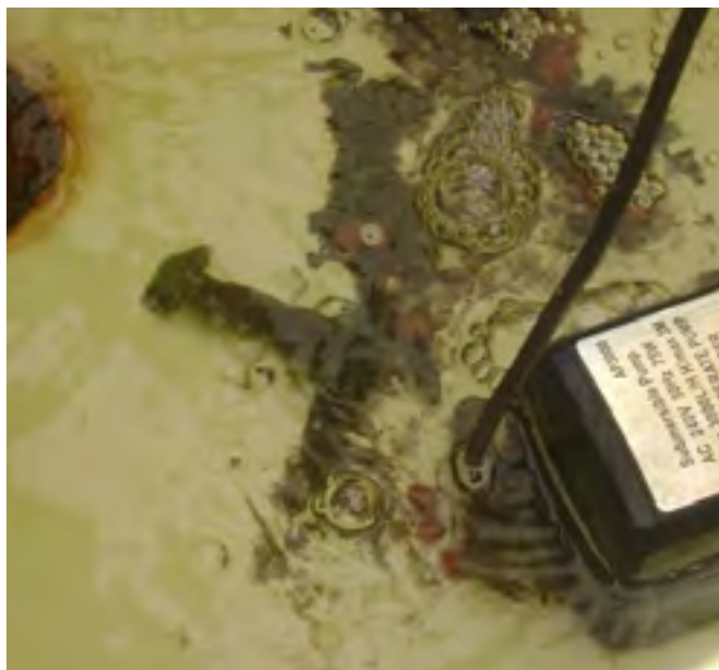
3000lph submersible pump
