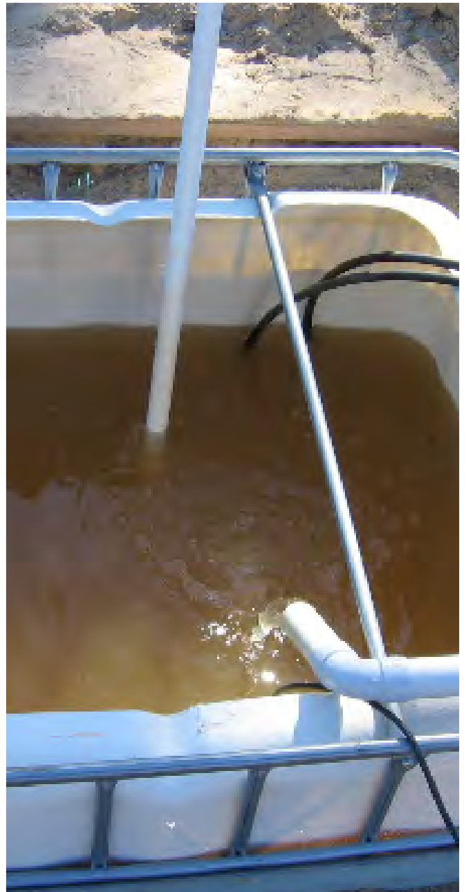
Sump tank buried and supported in ground
