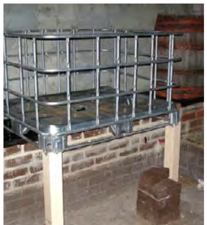
The metal base for the IBC is just deep enough that it can fit a 90 degree outflow pipe
