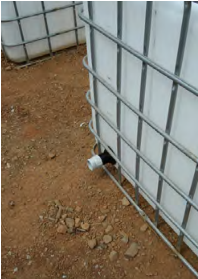
Tank fittings are one of the safest ways to plumb an IBC
