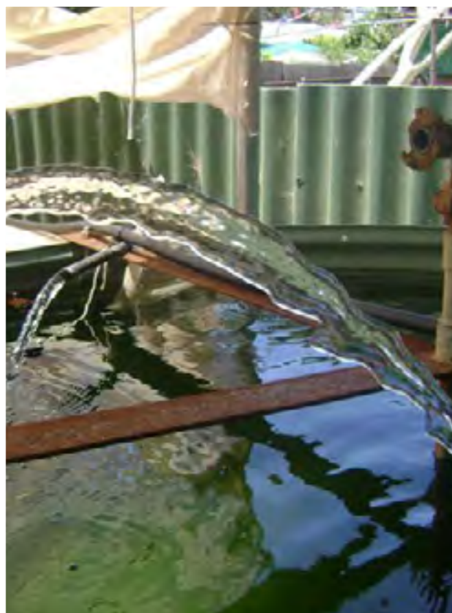
3000 litre rain water tank added to the system
