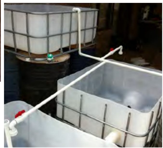
Irrigation line using 25mm pipe and ball valves
