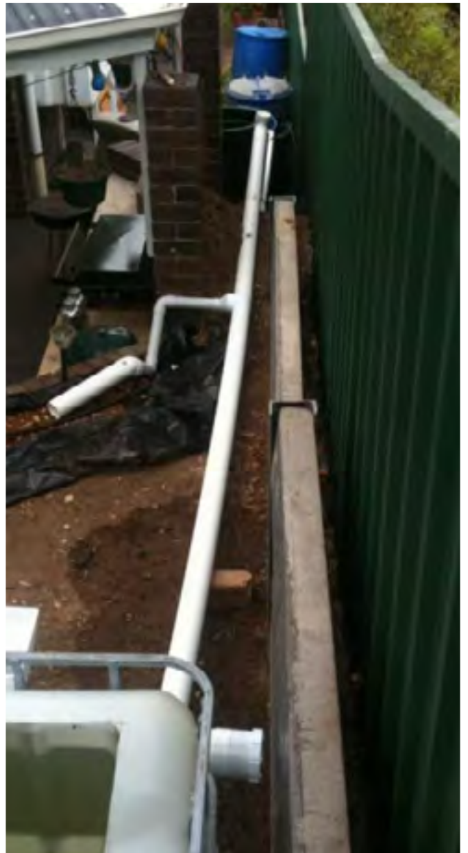
Side view showing where they are situated in the backyard. Home made level control skimmer boxes. 90 mm storm water PVC with removable ends for cleaning
