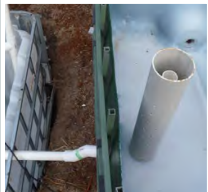
Details of the standpipe and media guard in the growbed, with the drain pipe coming out of the bottom into the sump
