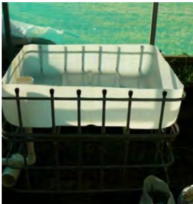
Not enough support for this bed when the gravel went in
