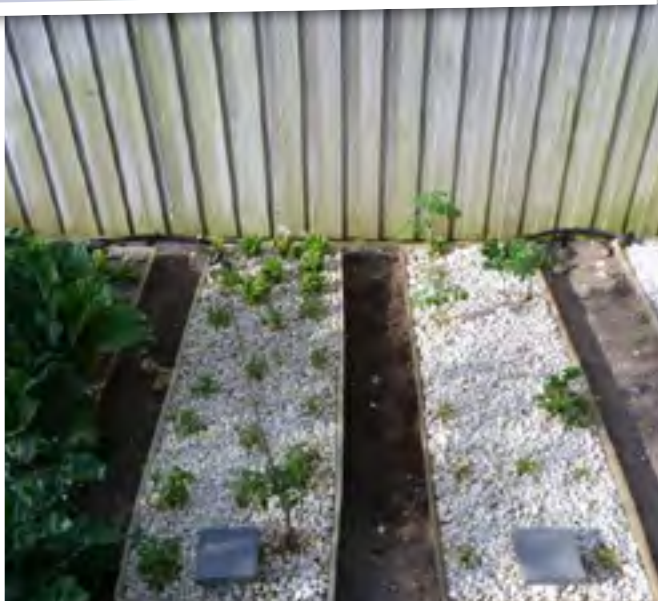
Growbeds installed at ground level and all drain pipes buried. Irrigation line runs along the fence behind
