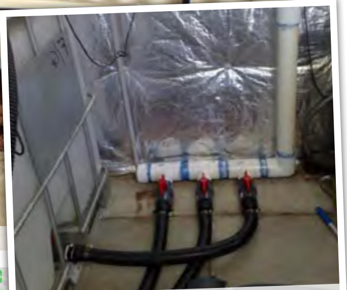
Piping from the IBCs heading out to the growbeds
