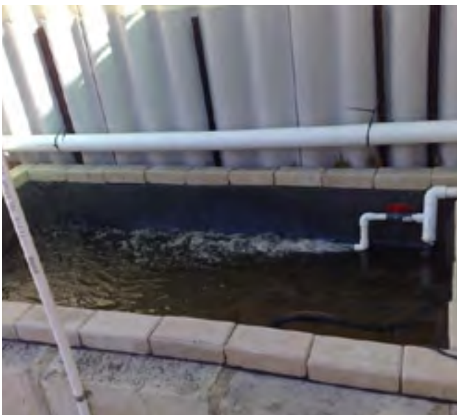
The main sump tank what contains the pump; Sumps all set up, stands partially buried to a better height
