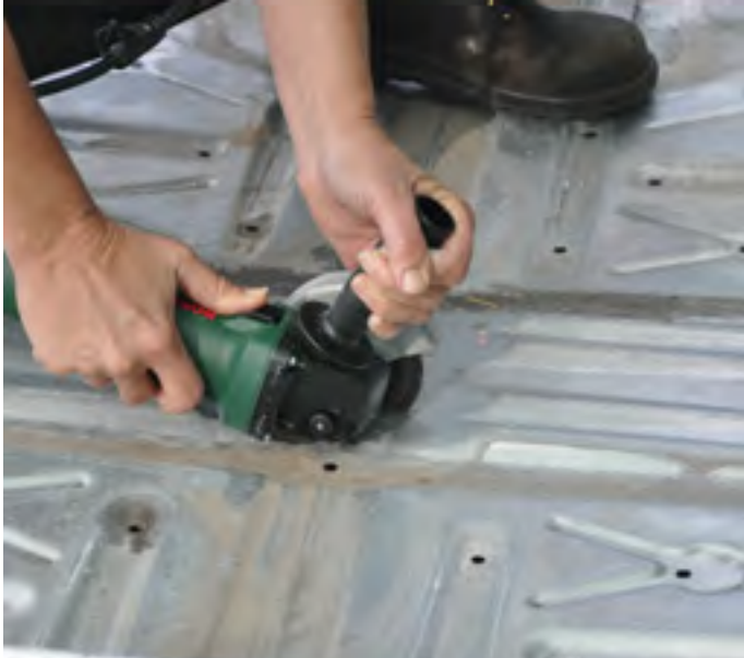
Cut the hole in the steel base large enough for the drain fittings
