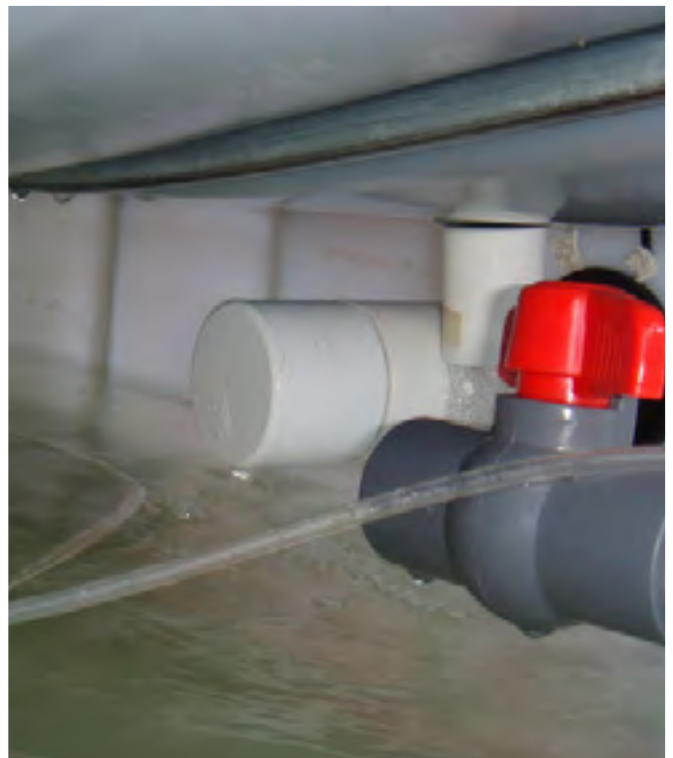
Piping and fittings under the bed
