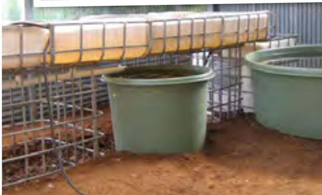
Once the beds are in place, the drain pipework can then be plumbed in
