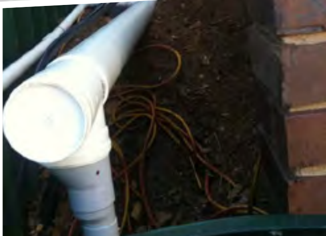
Looking from the filter and sump module
