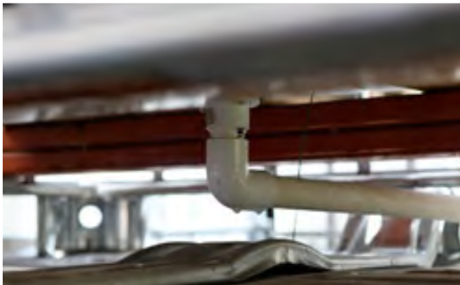
Early leaks in the systems plumbing needed fixing
