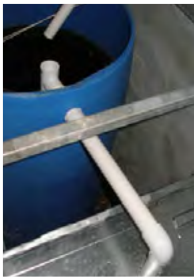
The plates on the IBC cage are the perfect size to use as lids for the two ends of the pond
