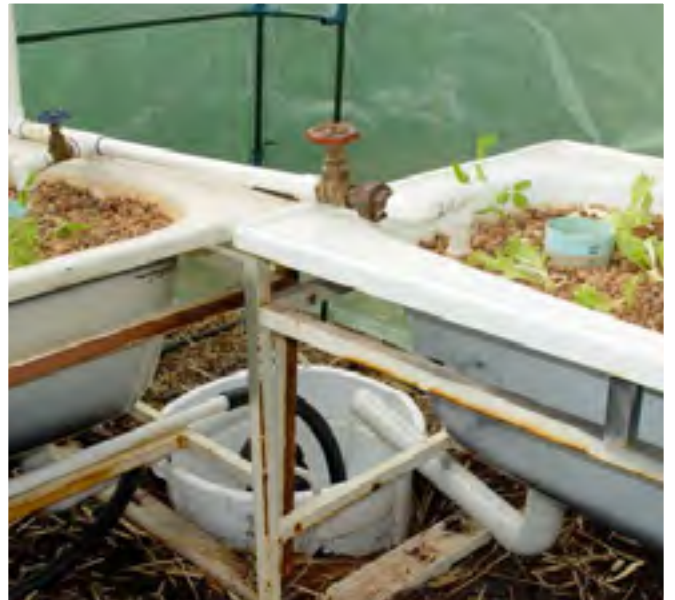
Inline taps are used to regulate the water distribution to the bathtubs
