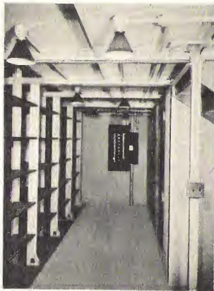
STACK LIGHTING SYSTEM
