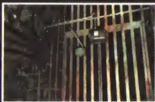
Closed circuit cameras, motion and heat detectors, alarm systems...
