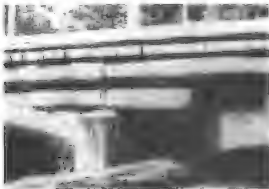
Fig. 4. Bridge girder over Kilcoy Creek, Conondale Ranges. The hibernaculum of Litoria pearsoniana was located in the arrowed crack.
