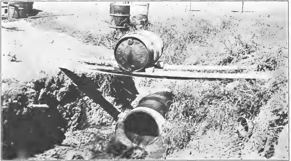
FIG. 65.—Oil drip at termination of storm sewer at Kelly Field, Tex.
