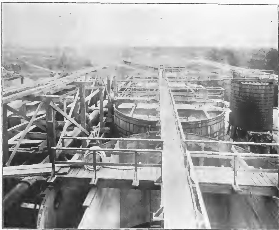
FIG. 36.—Coagulation and settling tanks, Camp Meade water-purification plant
