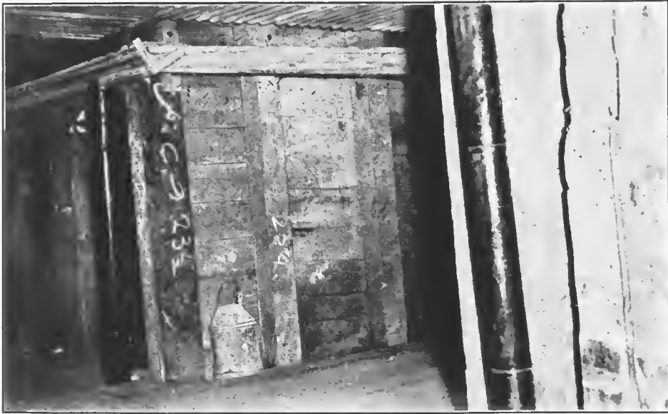
FIG. 16.—Interior of dugout built by American Engineers, at Boucq, Second United States Army area. Note the corrugated-iron ceiling which sheds seepage water into troughs which discharge into gutters under the floor
