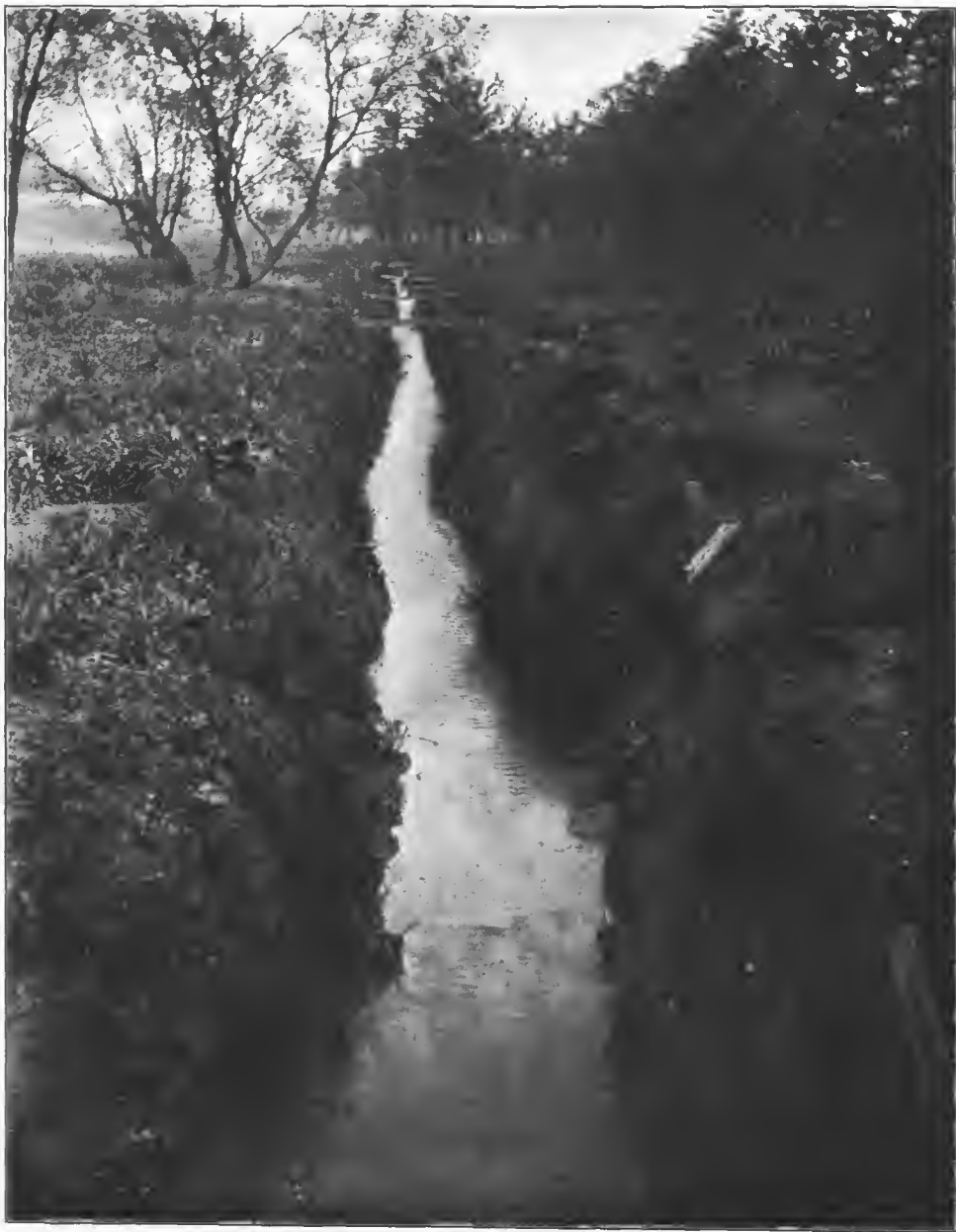
FIG. 60.—One of the early ditches dug by the construction quartermaster, Camp Meade, Md.
