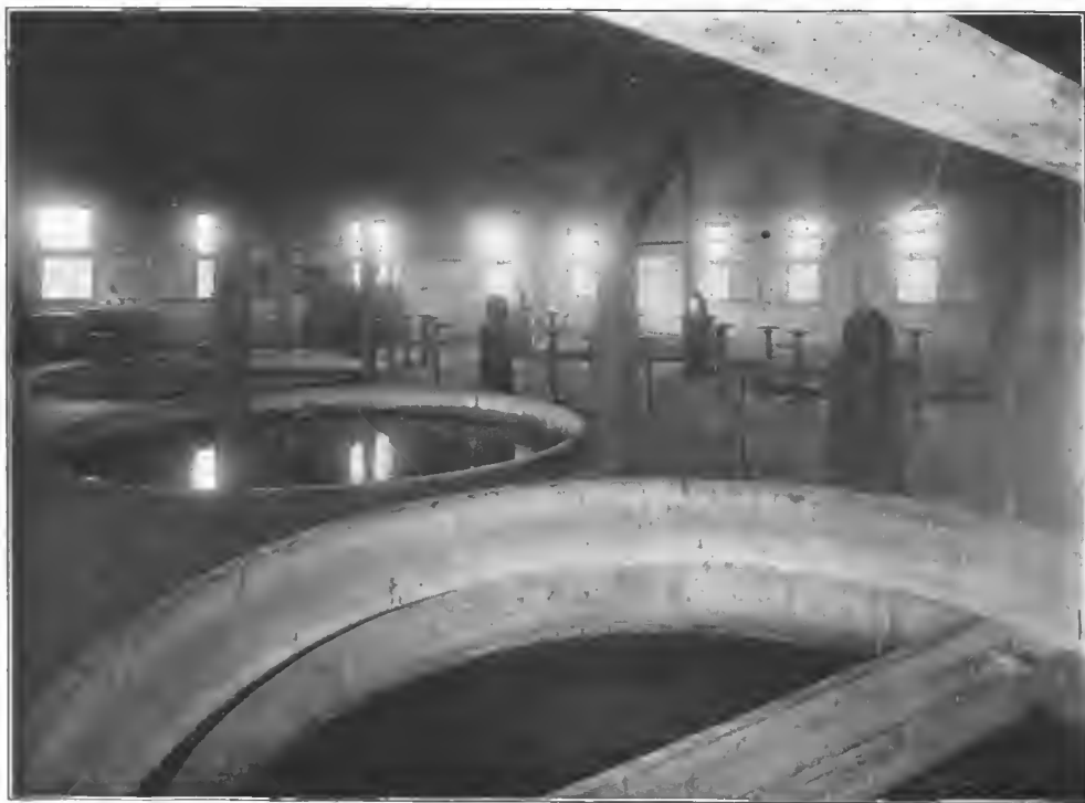
FIG. 38.—Filter room, Camp Meade water-purification plant
