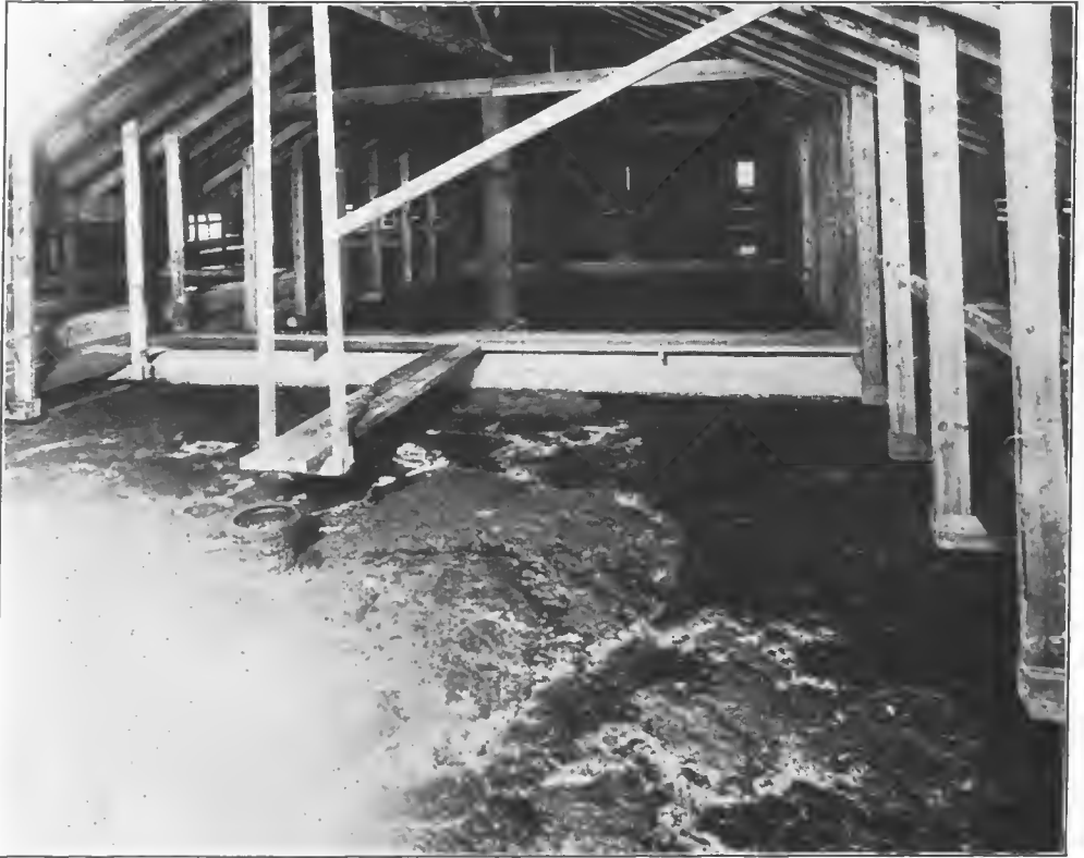
FIG. 41.—First compartment of typical Construction Division septic tank, showing scum formation, Camp Meade, Md.
