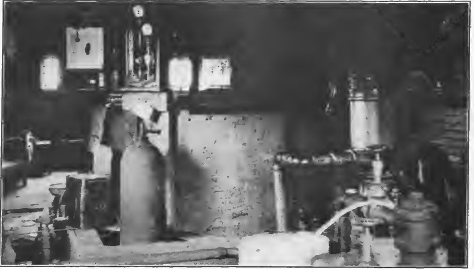
FIG. 57.—Euvezin water plant, American Expeditionary Forces. Interior of pump house, showing filter and chlorimeter
