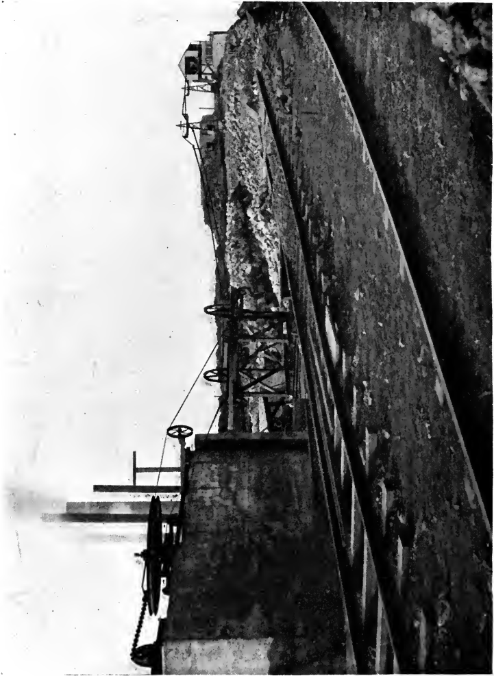
FIG. 91.—Installation at Middlesbrough : General View of Line.
