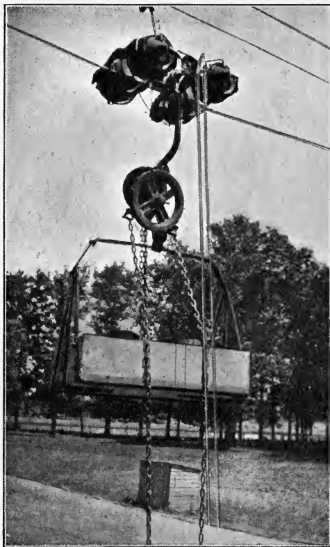
FIG. 136.—Installation on Telfer System : View showing Truck with Carrier and Hoist.
