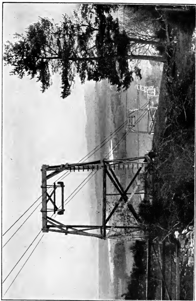
FIG. 120.—Installation at a Saw Mills in Scotland : View along the Line.
