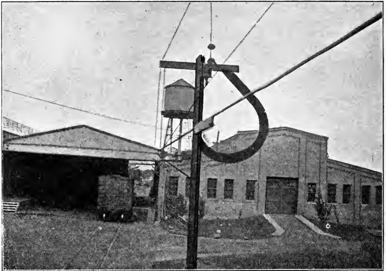
FIG. 135.—Installation on Telpher System : View at Works End of Line.
