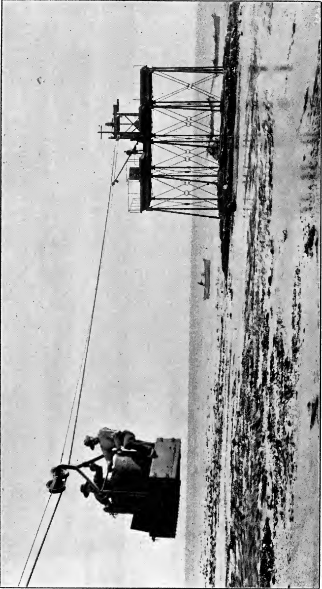
FIG. 131.—Installation as a Pier in South Africa: View of Sea Staging with a portion of Rope-Way and Carrier thereon.
