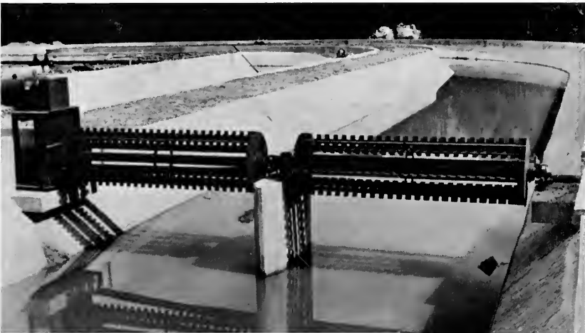
Cage rotors for a municipal oxidation ditch. Rotor covers are removed. (Photo courtesy of Lakeside Engineering Corp.) (Fig. 11)
