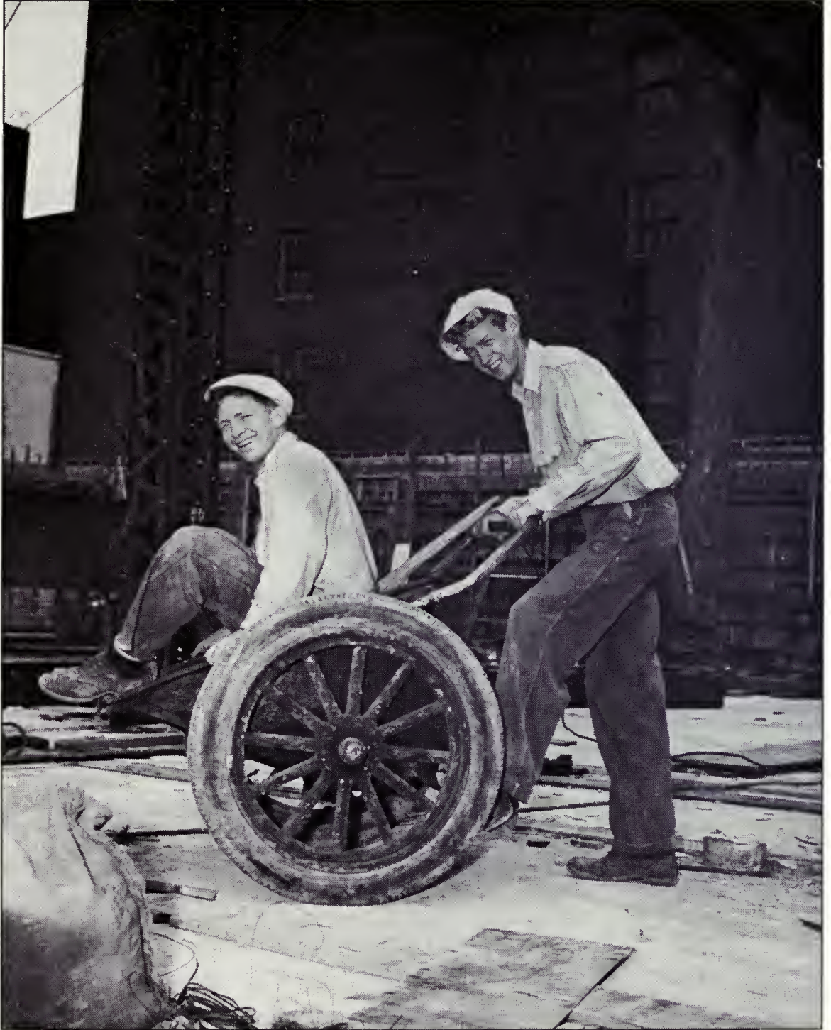
Duayne Gordon and George Maslach, University of California students in electrical and mechanical engineering, respectively, worked all summer of 1941 on the NBC Building, then returned to their studies.
