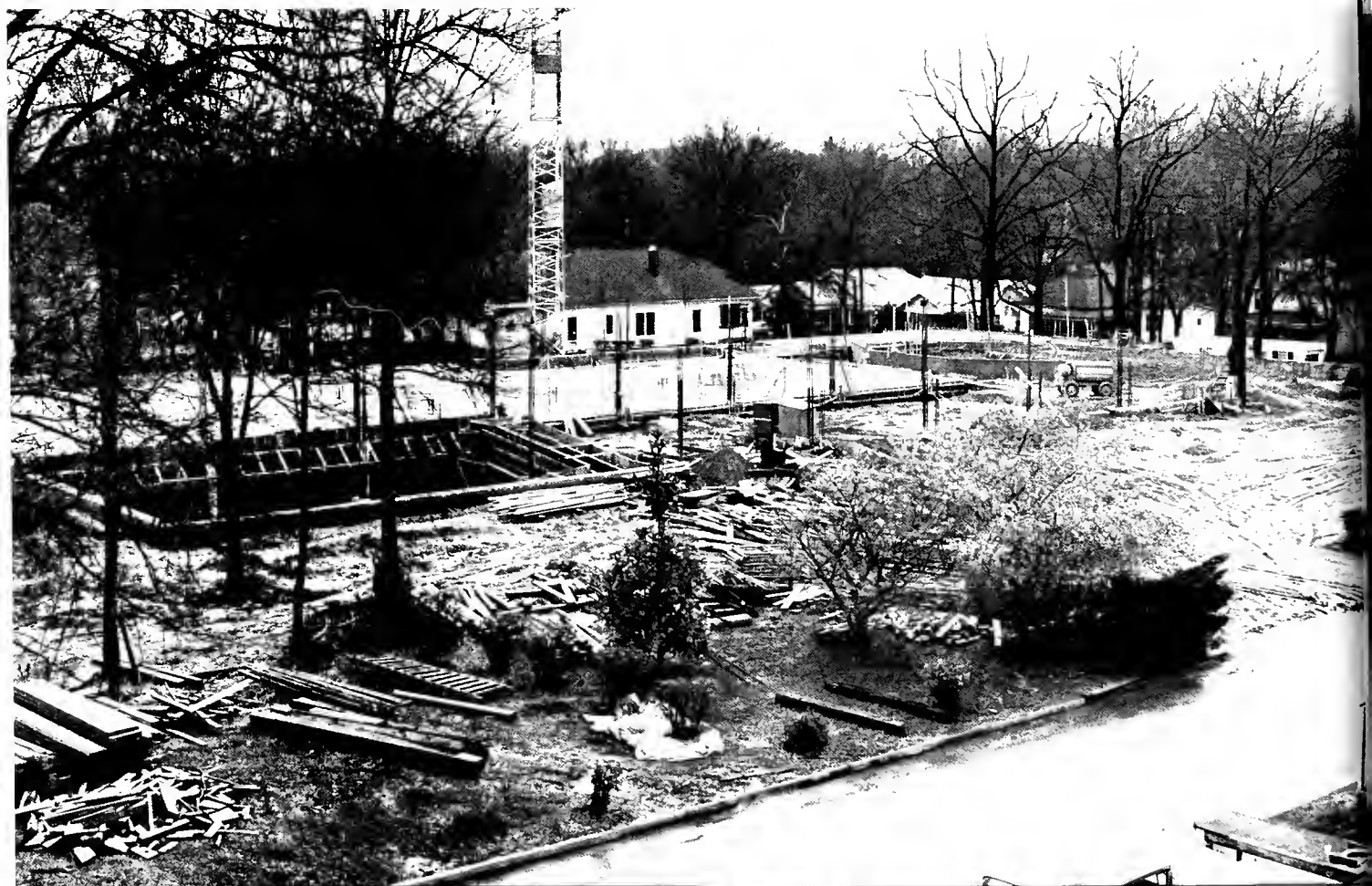
Early spring rains have made Georgia red clay mud at the site of the Dana Fine Arts Building.
