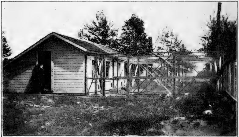
SCHOOL POULTRY HOUSE BUILT BY AGRICULTURE CLASSES AT GREEN BAY EAST SIDE HIGH SCHOOL.
