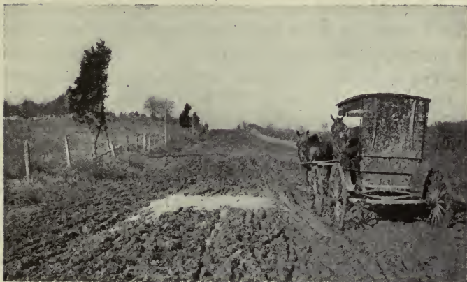
An earth road that needs improving.
