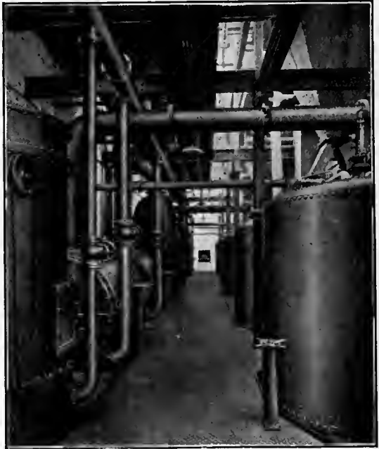
View of Solvent Extraction plant, capacity up to 1,200 tons per week of PALM KERNELS and many other seeds, making oil for margarine manufacture.
