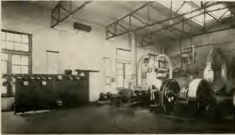
COLLEGE POWER PLANT
