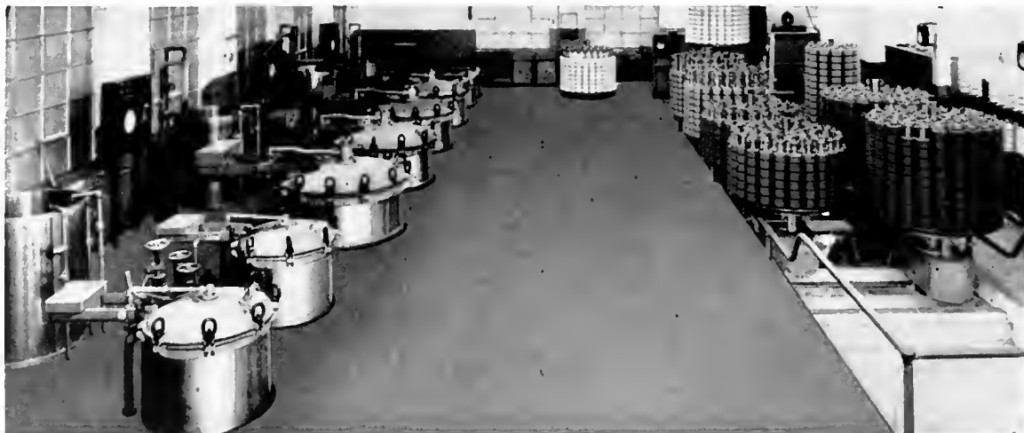
Recent installation of Gaston County "automatically controlled" Package Dyeing Machines, Extractor, and Dryers.
