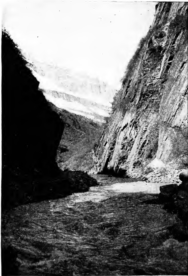
Heavy rock work under way in 1944 on Mile 2½ relocation of Richardson Highway, Mile 14½ from Valdez. (Courtesy Ike P. Taylor.)
