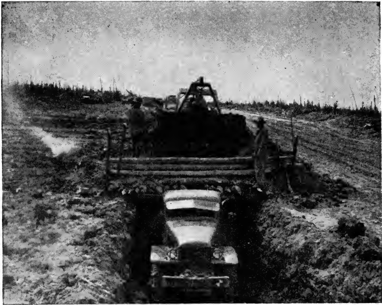
A novel system of loading dirt in the absence of shovels. The truck backs into the depression and is loaded from above by a bulldozer.
