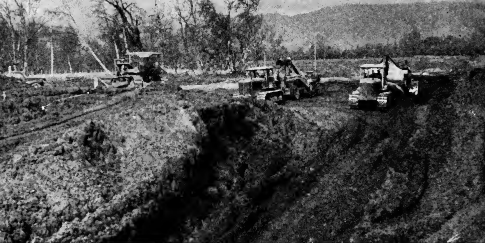
Grading on the Glenn Highway, Mile 3 from Palmer—a relocation of the old road. (Courtesy Alaska Road Commission.)
