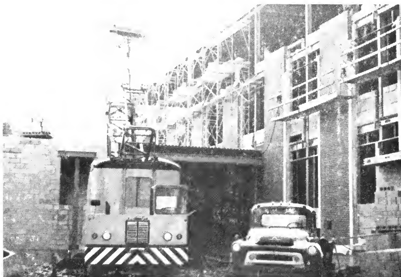
Construction on Science Complex continues to move along, with completion scheduled for September, 1966.
