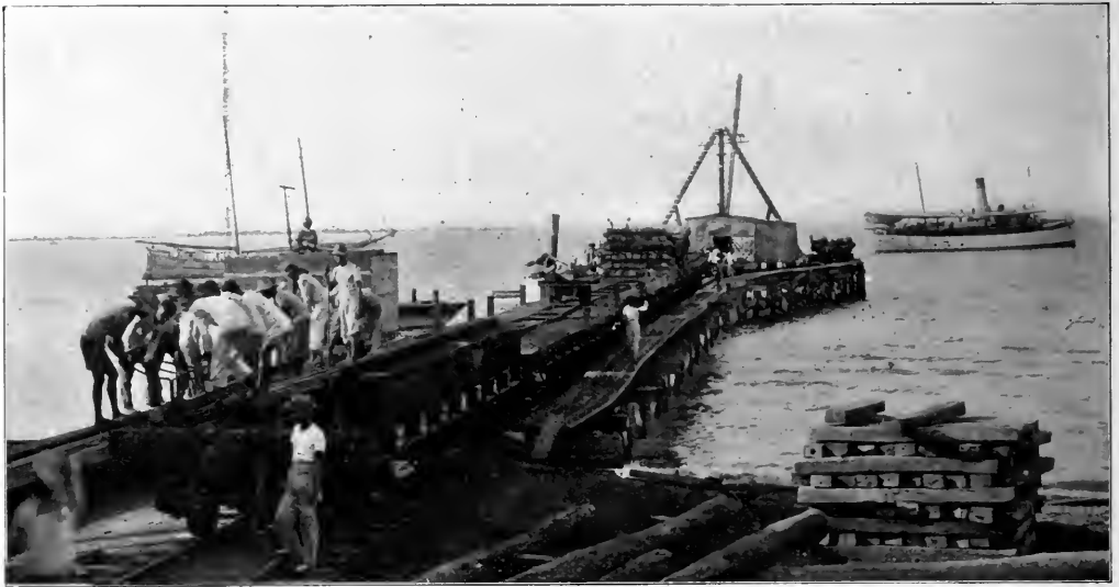
NATIVES LOADING RAILS ON TRACK-LAYING CARS ON THE TEMPORARY WHARF IN CEBU
