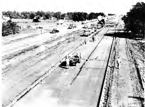
Typical photograph showing dual pavers in operation, U. S. Route 66 south edge of Farmersville, Montgomery County.
