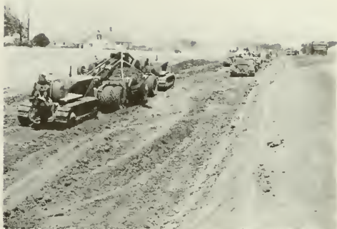
Heavy grading equipment making grade change, U.S. Route 51 north of Vandalia, Fayette County.
