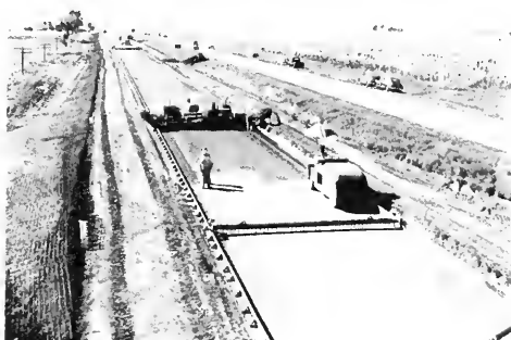
Typical photograph of subgrade preparation before placing concrete, U. S. Route 66 south of Farmersville, Montgomery County.
