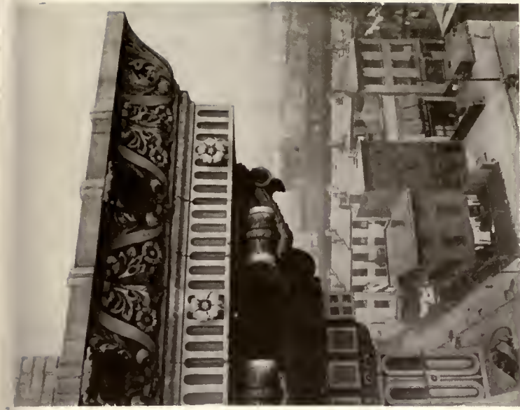
BROOKLYN ACADEMY OF MUSIC. Herts & Tallant, Architects. Section of main cornice of polychrome terra-cotta.
