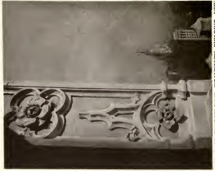
DETAIL OF WINDOW-JAMB, WOOLWORTH BUILDING, NEW YORK. Cass Gilbert, Architect. Polychrome terra-cotta.
