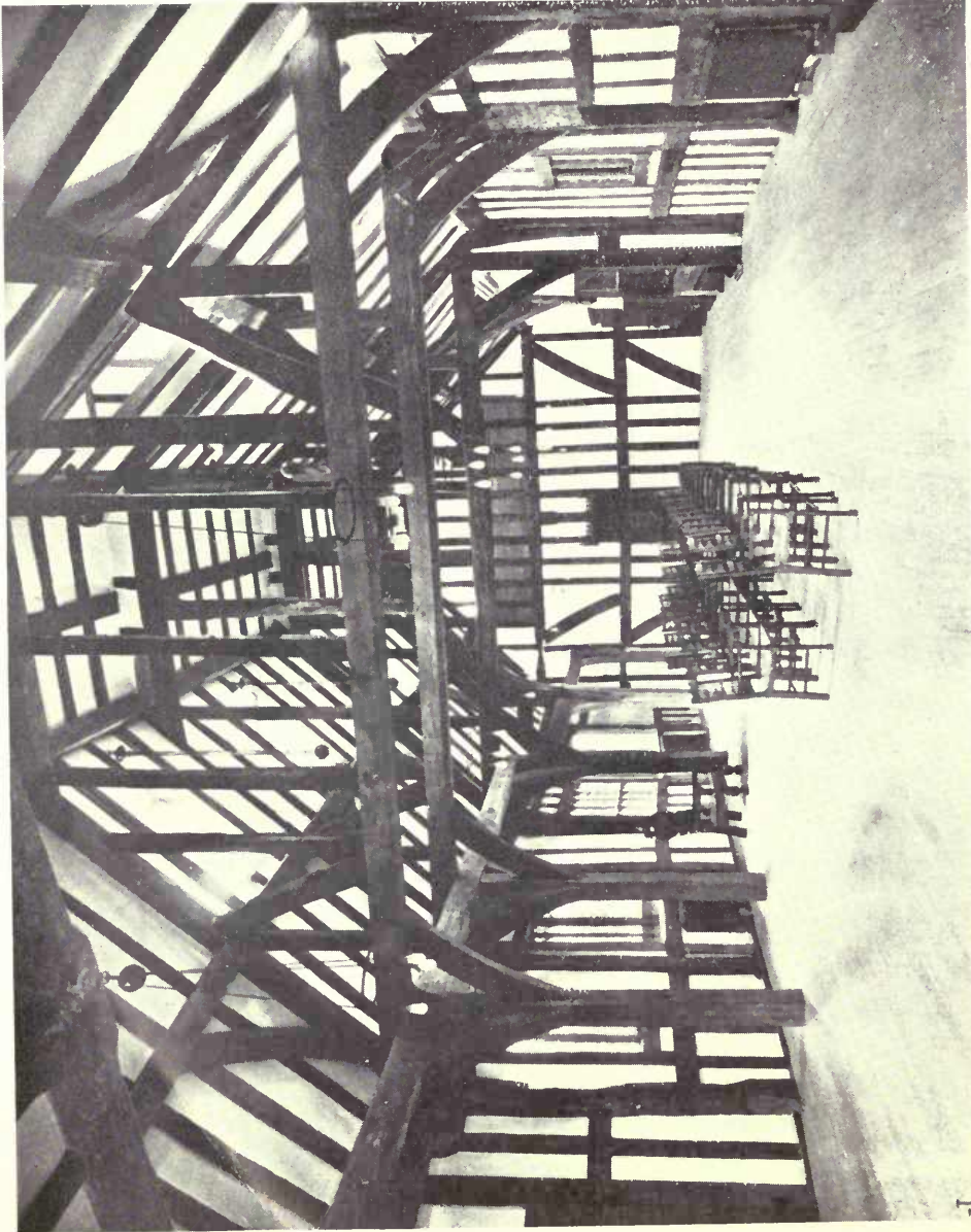
Restoration of St. William's, York. Northern Convocation House: House of the Vicars Choral. TEMPLE MOORE, Architect.
