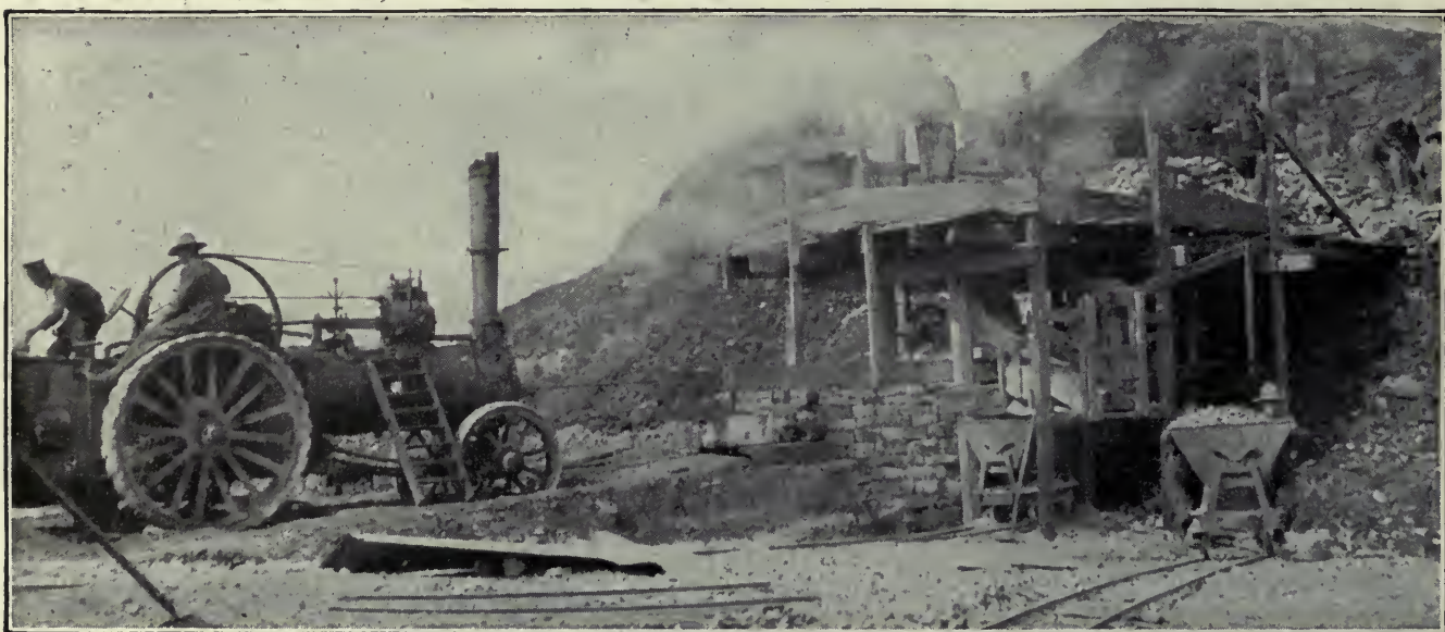
THIS QUARRY, TAKEN OVER FROM FRENCH, IS SHOWN PARTLY EQUIPPED WITH GYRATORY CRUSHER, THE OVERHEAD STORAGE BINS NOT HAVING BEEN BEGUN
