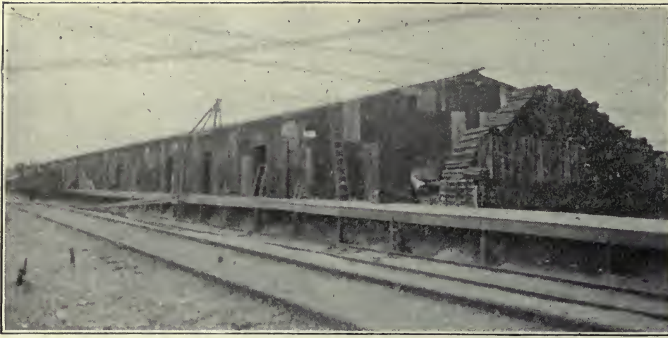
B. AFTER THE WOODEN FRAMEWORK WAS SET UP THE BUILDINGS WERE SHEATHED AND ROOFED WITH CORRUGATED IRON
