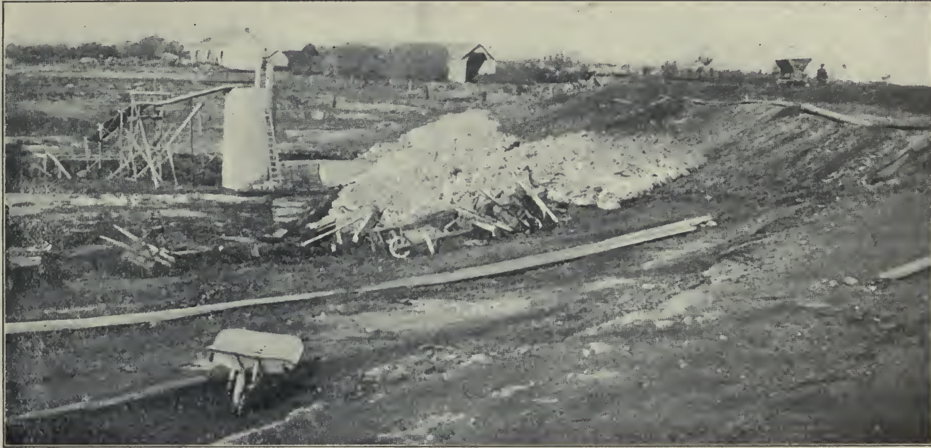
THIRTY-THOUSAND YARD EARTH DAM AT FRENCH SEAPORT BUILT WITH PICK AND SHOVEL
