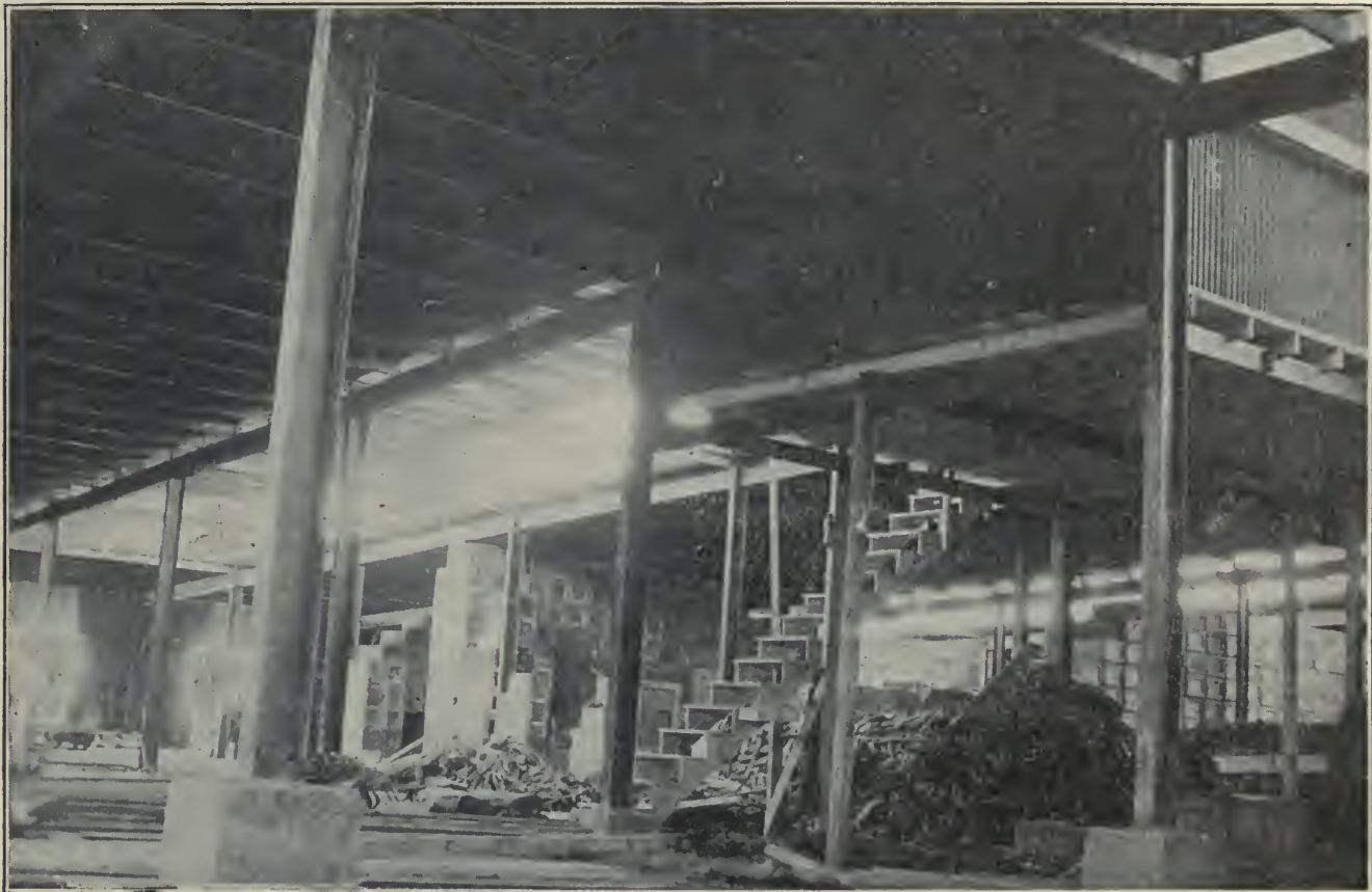
G. INTERIOR OF FINISHED ORDNANCE STORAGE BUILDING—COLUMNS SUPPORTED ON CONCRETE FOOTINGS OF DIFFERENT HEIGHTS TO GIVE SLOPE TO ROOF, SINCE ALL COLUMNS ARE OF SAME LENGTH
