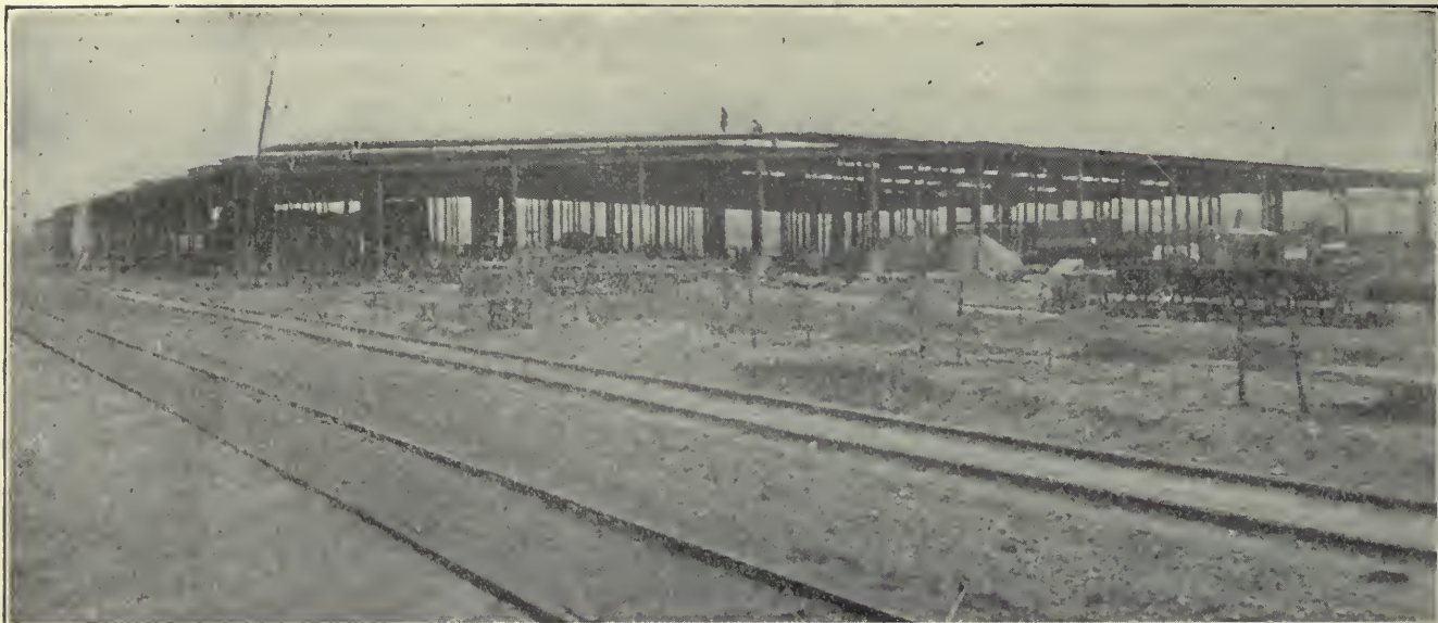
E. HOW ONE OF THE STEEL-FRAME ORDNANCE BUILDINGS, THE MACHINE SHOP, LOOKED ON APRIL 5
