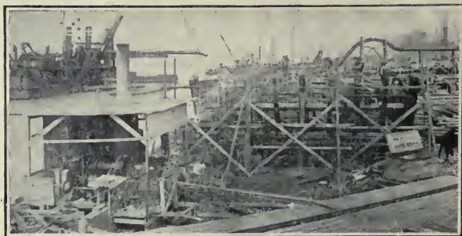
D. DREDGE PUMPING SAND FROM SCOW TO MAKE RAILROAD FILL—NOTE END OF ELEVATED PIPE LINE AT RIGHT, THROUGH WHICH SAND IS PUMPED
