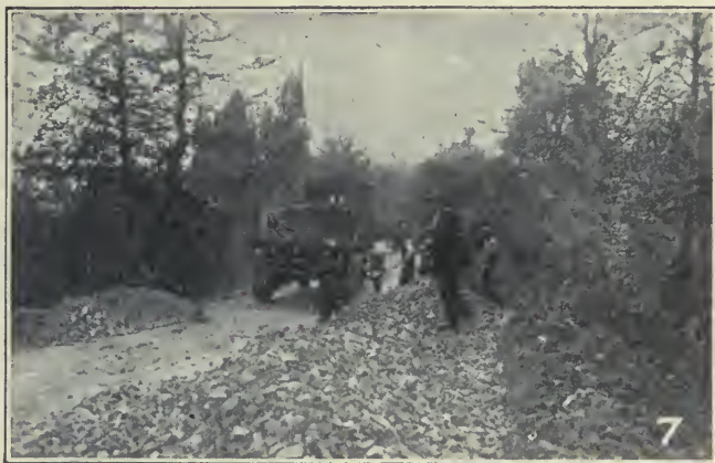
FIG. 6, 7 AND 8. WIDENING A NARROW ROAD LEADING INTO AN IMPORTANT AMERICAN ARMY CAMP — MOTOR TRUCKS DELIVER CRUSHED STONE TO THE JOB, AND THE STONE IS SPREAD ON EITHER SIDE OF THE ORIGINAL ROAD
