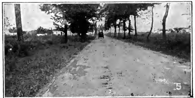
FIG. 5. FRENCH ROAD OF "GRANDE COMMUNICATION" TYPE—USE BY ARTILLERY IS PRODUCING RUTS AND HOLES WHICH WILL SOON NEED ATTENTION
