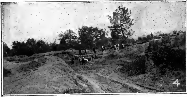
FIG. 4. SAND AND GRAVEL PIT BEING WORKED BY SPANISH LABOR, DIRECTED BY A DETAIL OF ONE OF OUR ROAD-BUILDING REGIMENTS
