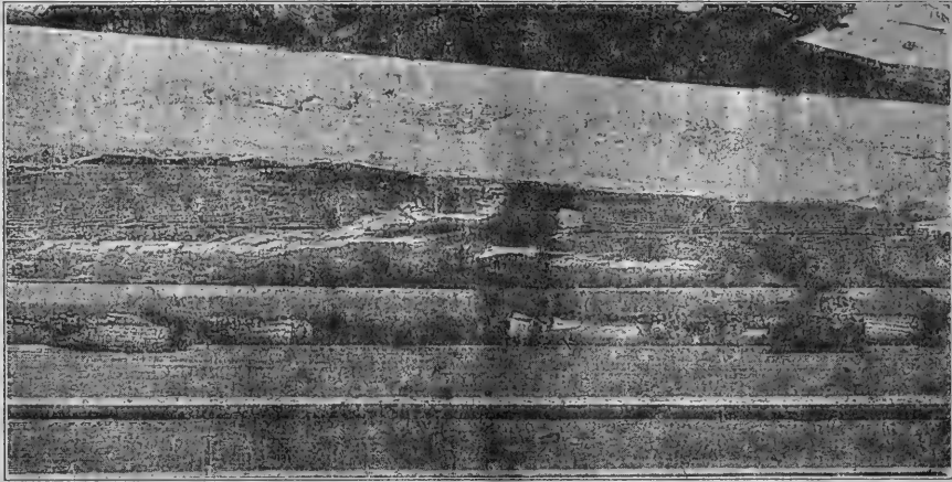
Decayed Lumber in a Corn Crib (Courtesy U. S. Forest Service)
