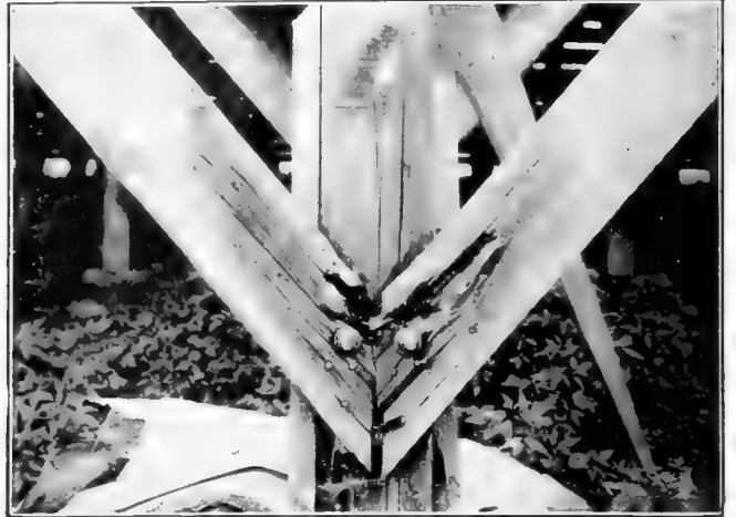
Decay in braces at joint where moisture tends to collect. (Courtesy of U. S. Forest Service)
