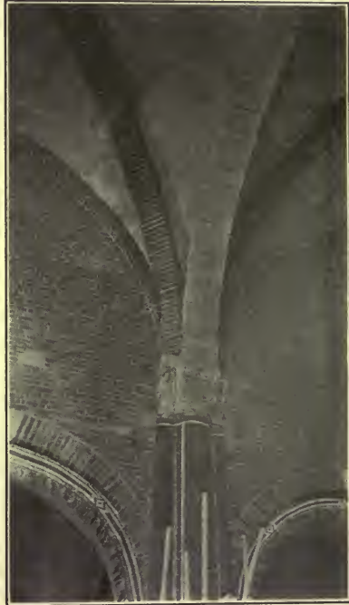
FIGURE 1.—DETAIL OF CLEARSTORY ABOVE THE EASTERNMOST ALTERNATE PIER ON THE NORTH SIDE OF THE NAVE.
