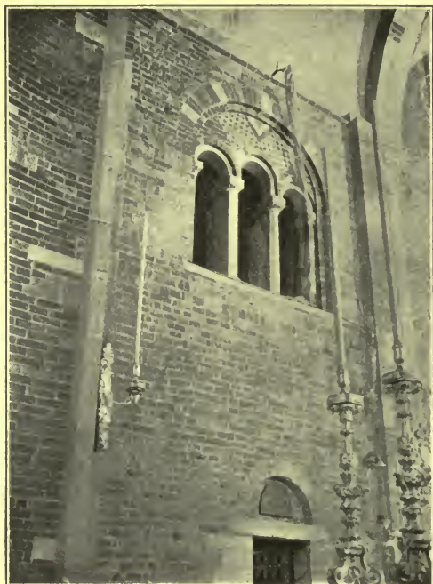
FIGURE 3. — SOUTH WALL OF CHOIR; SHOWING BARREL VAULT AND FRAGMENTS OF ANCIENT MASONRY.
