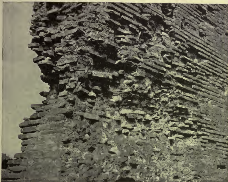
FIGURE 1.—A REFACED WALL. 1
