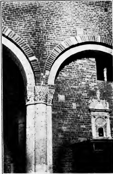
FIGURE 2. — EASTERNMOST PIER ON THE SOUTH SIDE OF THE NAVE ; SHOWING BASE AND PRE-EXISTING CAMPANILE.
