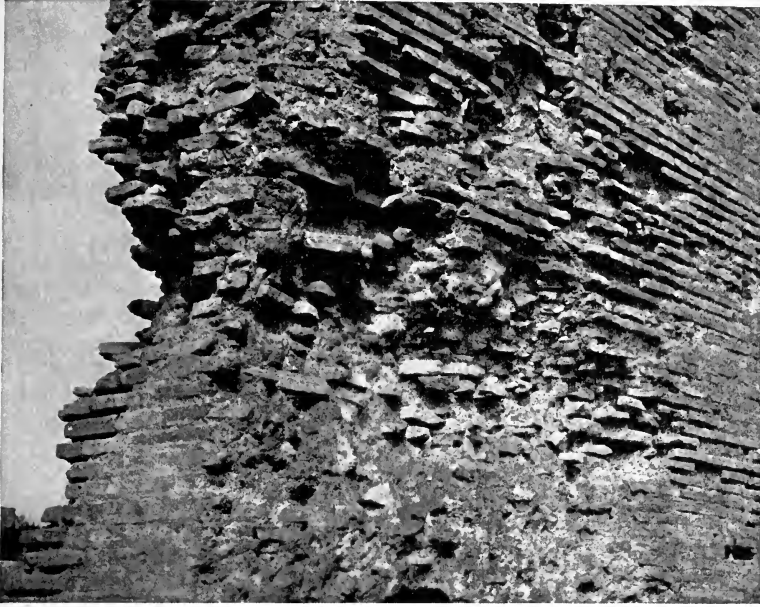
FIGURE 1.—A REFACED WALL. 1
