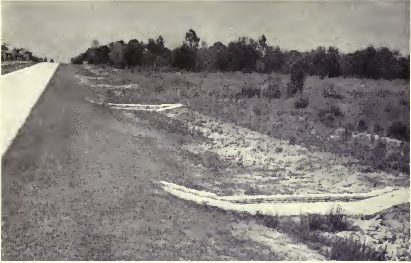
Strip sodding and seeding to control slope erosion on a Federal-aid Highway in Oxford County, Maine Courtesy Bureau of Public Roads
