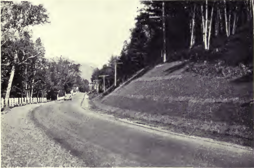
Ditch checks prevent erosion on one of Florida's highways Courtesy Bureau of Public Roads
