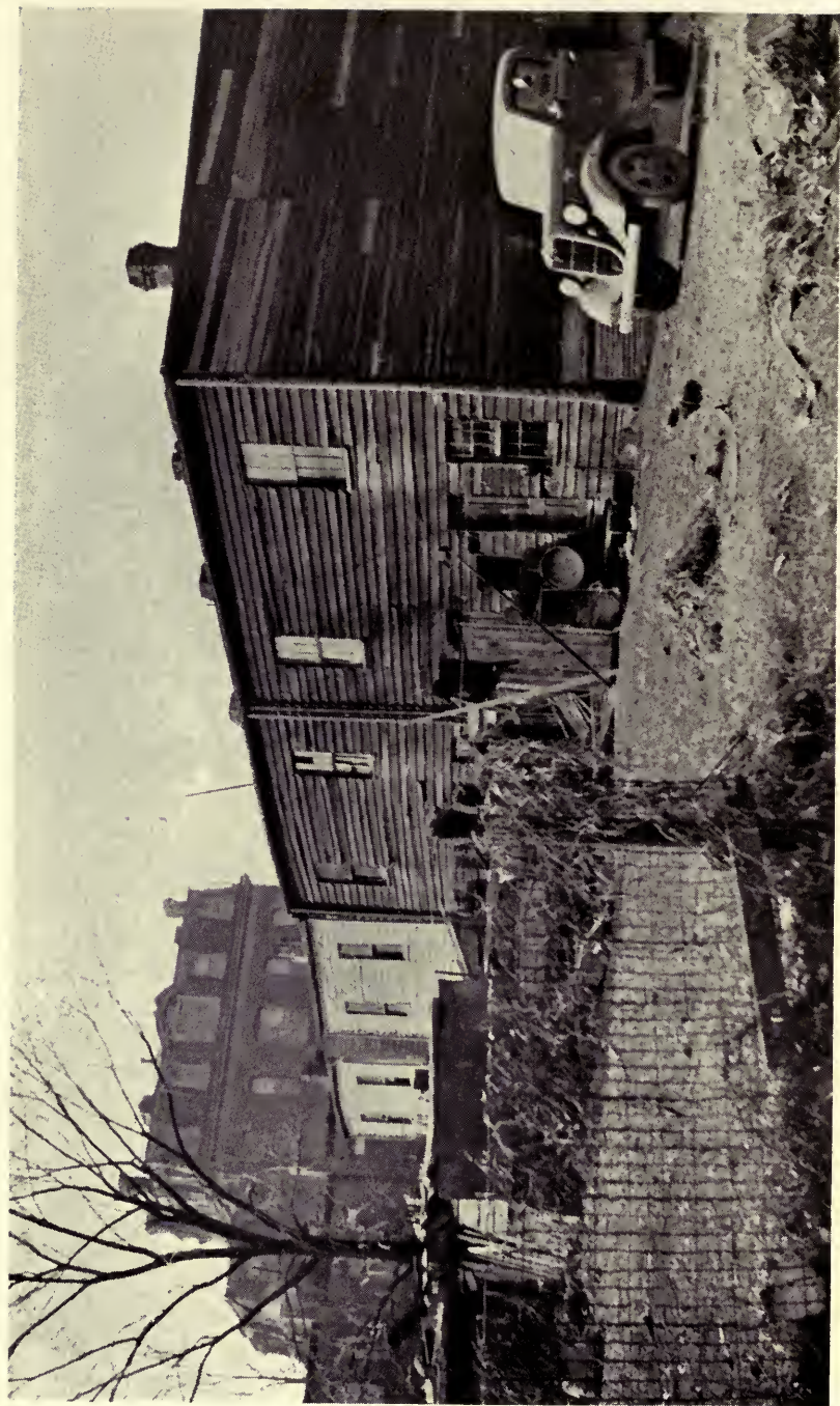
Dilapidated wooden alley houses located in the square immediately west of the apartment development. These houses are being acquired by the Authority and soon will be demolished to make way for a more effective development of the land they occupy. Courtesy Alley Dwelling Authority
