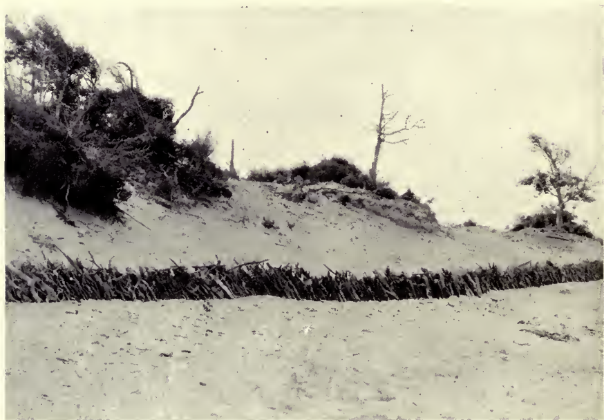
Sand fence constructed by WPA in beach erosion control Courtesy U. S. Department of the Interior
