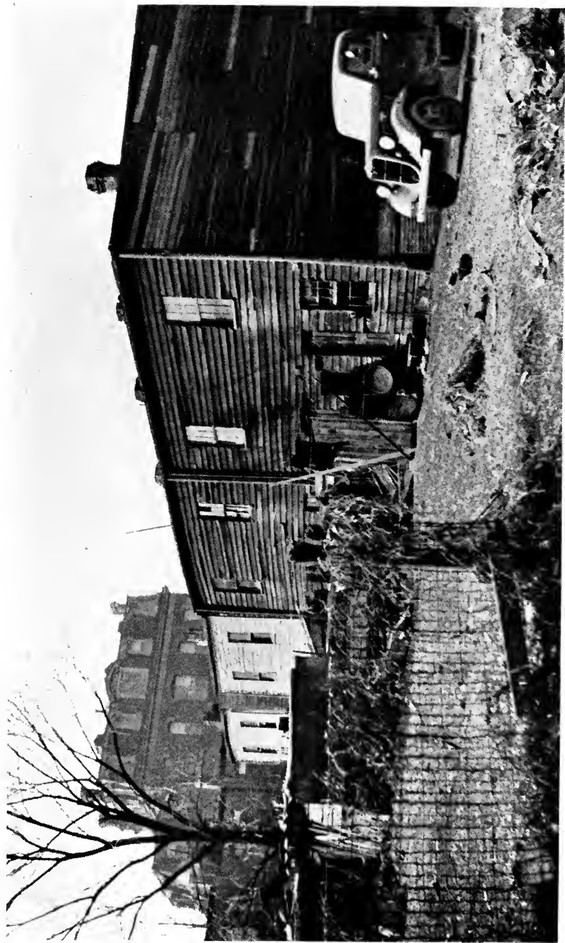
Dilapidated wooden alley houses located in the square immediately west of the apartment development. These houses are being acquired by the Authority and soon will be demolished to make way for a more effective development of the land they occupy. Courtesy Alley Dwelling Authority
