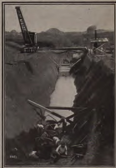
Photograph by the Pictorial News Co. EXCAVATING FOR THE CORE OF THE MIRAFLORES DAM.
