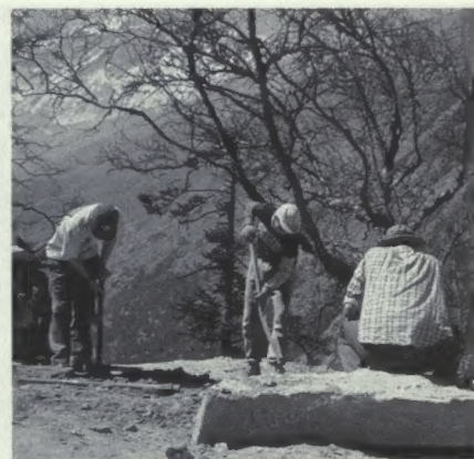
On the grounds of the Monastery digging for rocks that could be used to construct stairs.
