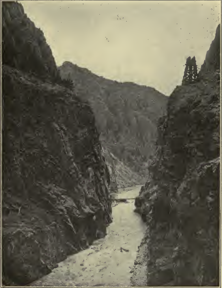
PLATE VIII.—Site of Shoshone Dam, Wyoming, looking up-stream. Under construction. Height from foundation to coping 310 feet. It will be the highest dam in the world.
