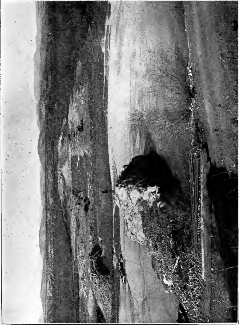
PLATE VII.—Site of Leashburg Diversion Dam on Rio Grande. Under construction. Canal gates will be set in Penasco Rock in foreground. Concrete dam will extend from Penasco Rock to join embankment in distance.
