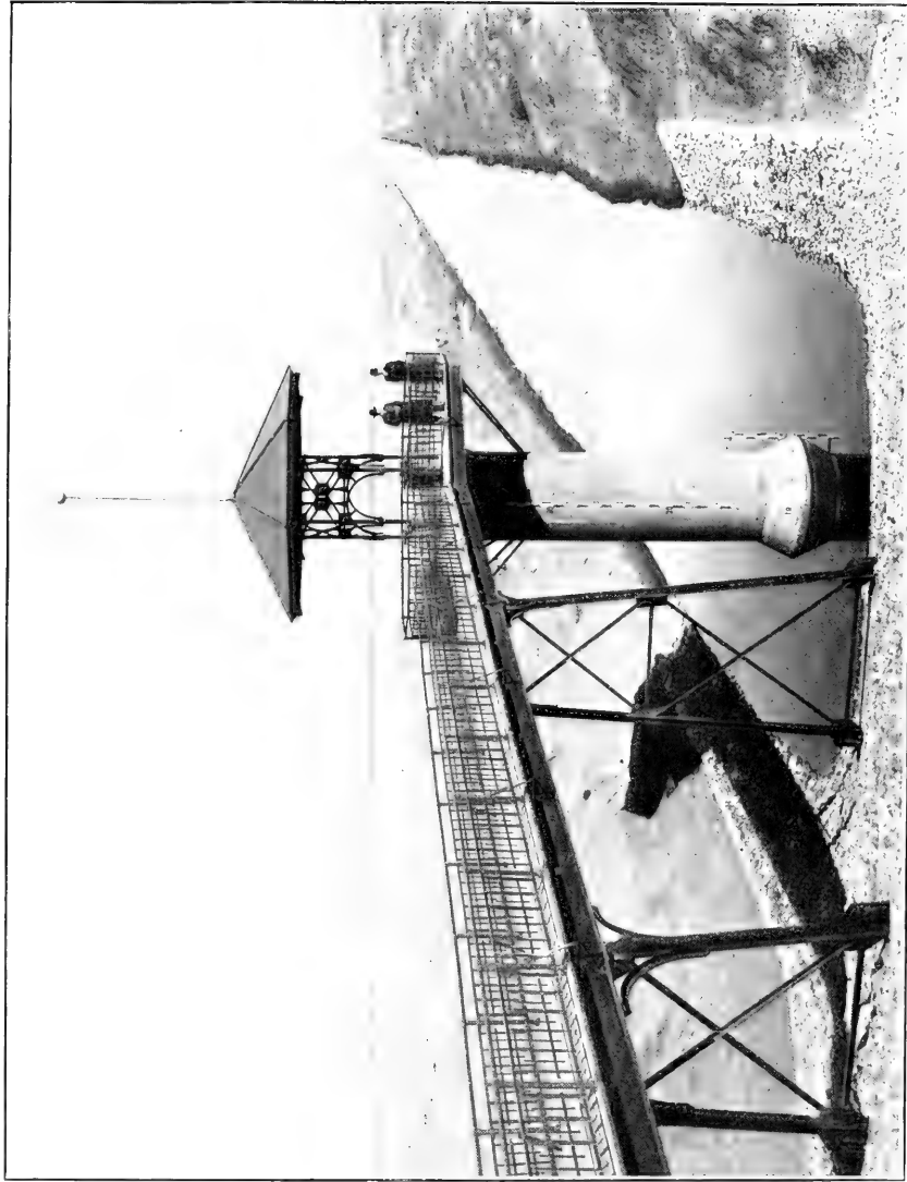
HONDO PROJECT, NEW MEXICO. HONDO RESERVOIR, LOOKING NORTH FROM OUTLET TOWER. (W. B. Lubken, January 31, 1907.)
