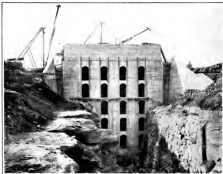
ASHOKAN RESERVOIR—UPPER GATE CHAMBER. Through this chamber the flow of water to the aqueduct will be regulated.
