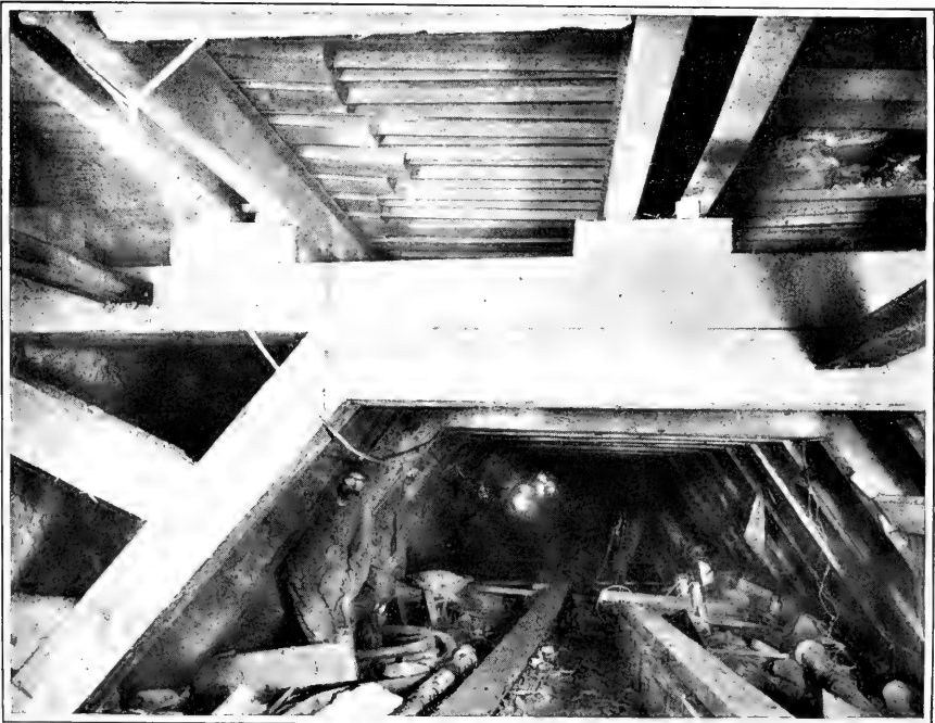
PERMANENT CHANNEL IRON SUPPORT FOR A TREACHEROUS ROOF. THE BEAMS WILL BE IMBEDDED IN THE CONCRETE LINING.
