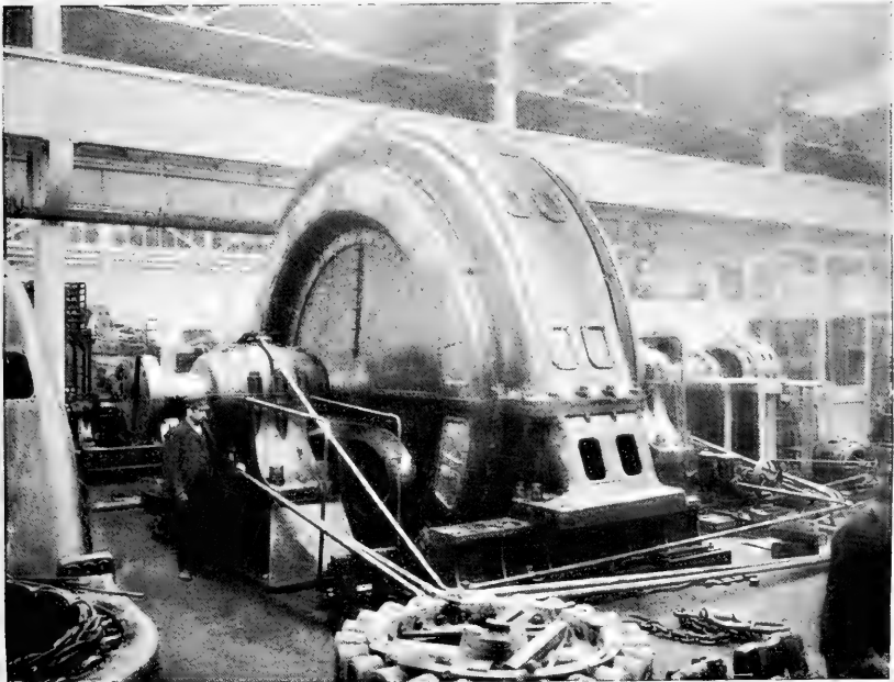
FIG. 2.—RJUKAN POWER HOUSE.
