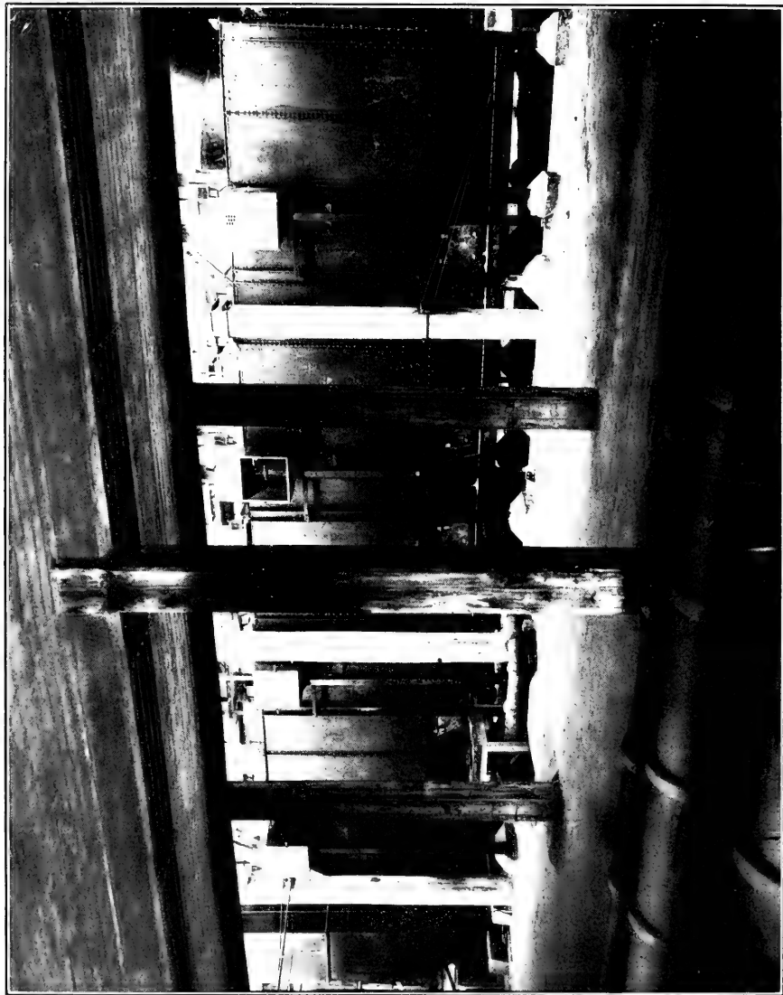
FIG. 40.—PRECIPITATOR AT HOOKER ELECTROCHEMICAL CO., SHOWING INSULATOR SYSTEM.
