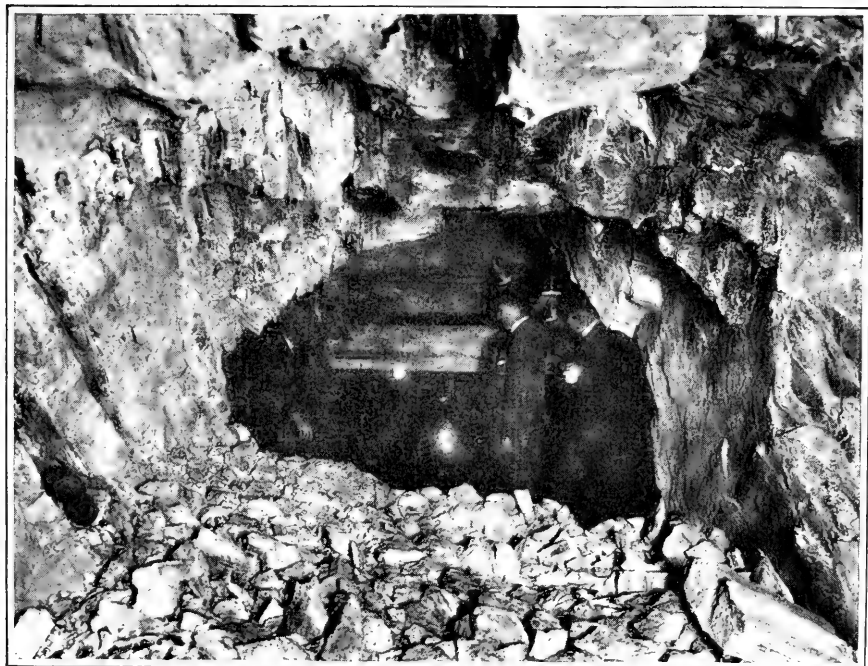
"HOLED THROUGH" FROM SHAFT 16 TO SHAFT 17. DANGEROUS ROCK OVERHEAD DUE TO VERTICAL SEAMS.
