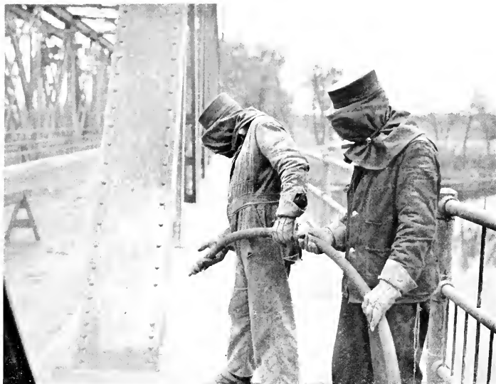
Painting is a necessary part of the City's bridge maintenance activities. Wearing protective masks workmen are shown sandblasting a bridge in preparation for painting
